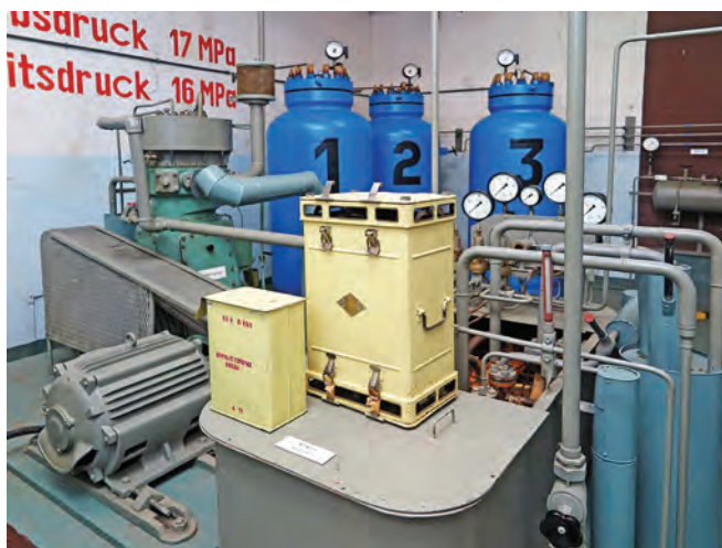
Stored air tanks and both parts of the portable combined Oxygen generator/CO2 scrubber. Photo Clive Penfold
